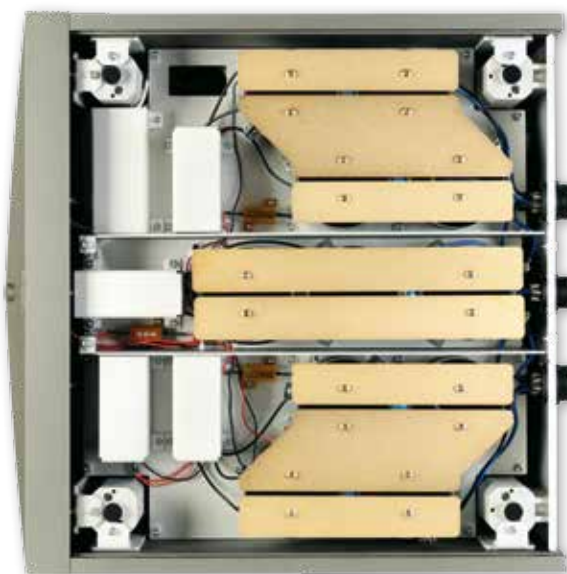
ABOVE: Supply unit includes three AC mains transformers/three banks of electrolytics for the IR LED PSU [centre] and Eq PSUs [top/bottom]
